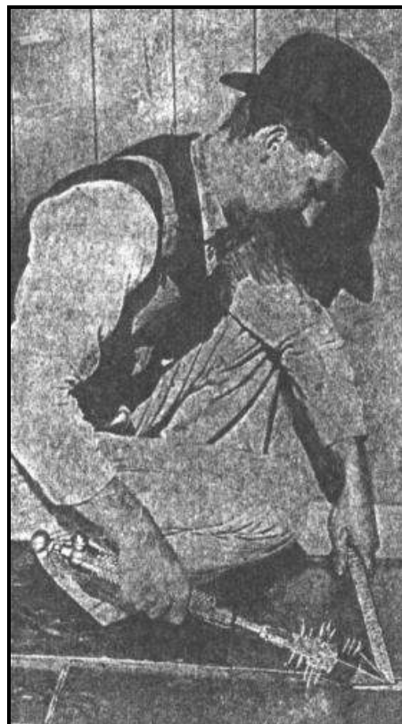
Worker using an Emmelmann Co. soldering iron on a sheet metal roof.
